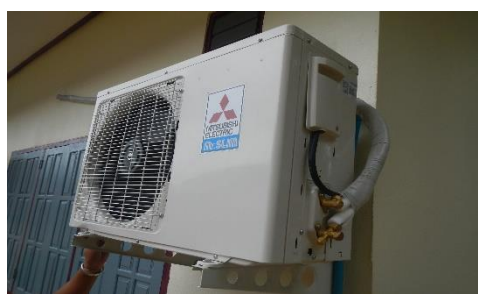
AC unit to improve air quality in the computer room
