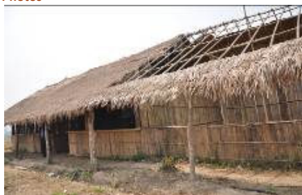
Temporary building with a barely intact roof
