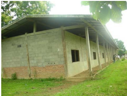
Never finished and unsafe !
