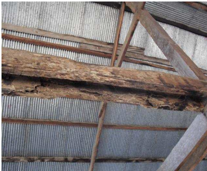
Rotten wooden roof beams
