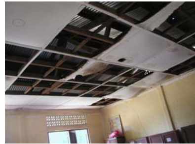
The leaking roof
