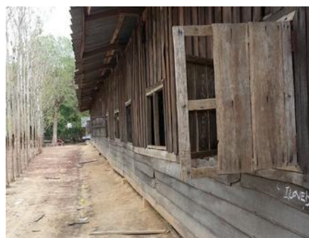
The school building is in disrepair
