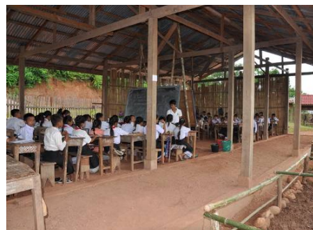
Classrooms with no walls
