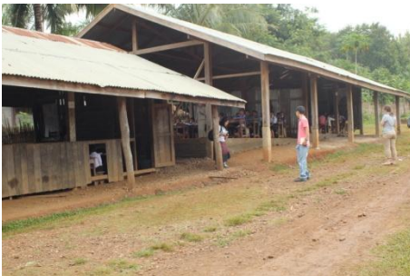
The temporary wooden building is not offering the students a good learning environment and poses security and health risks.
