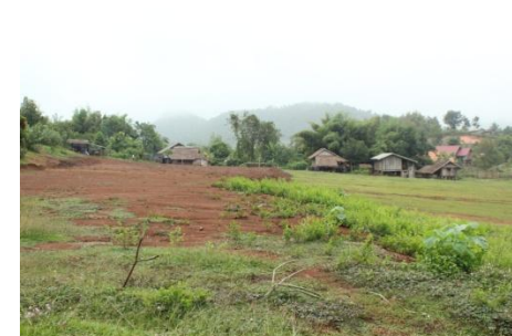
The community has already started filling in soil in preparation of the new construction site.
