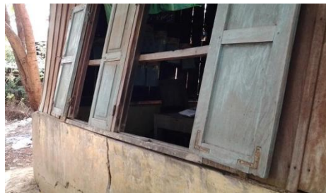
The walls are leaning and might collapse anytime
