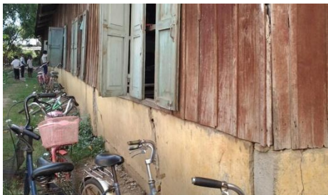
Deteriorating and unstable concrete foundation
