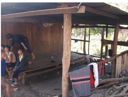
...in very bad condition and no longer safe
