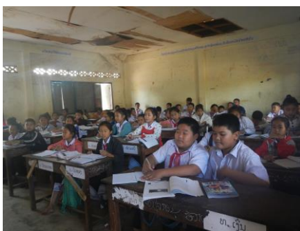
Some classrooms are visibly deteriorating
