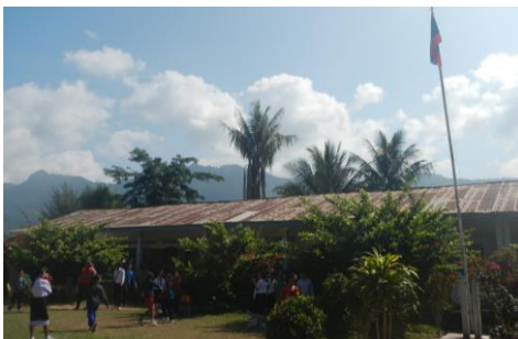
Made out of wood, this school building is starting to falling apart
