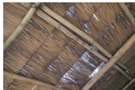
The building requires constant repairs in order to remain functional
