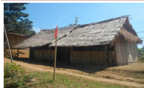
The buildings are unsafe and require constant repairs
