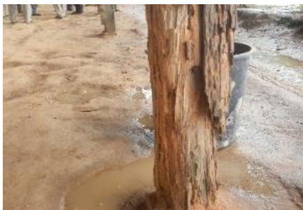
Age and termites have weakened the structures of the wooden building dramatically, making it dangerous for the students to use
