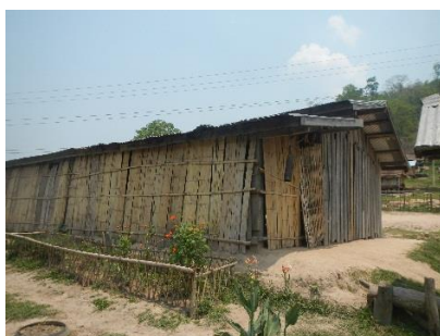
The school buildings are made of bamboo, grass and zinc roofs and are deteriorating rapidly
