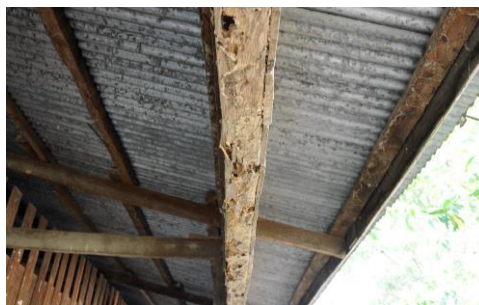
Termites have infested the wooden structures of the school building, rendering it unsafe
