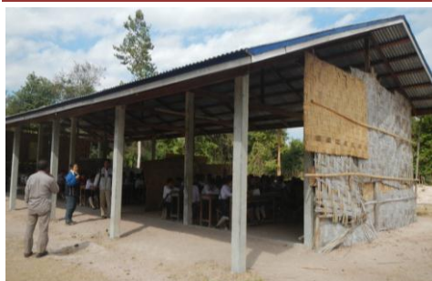
The school building offers no protection against rain
