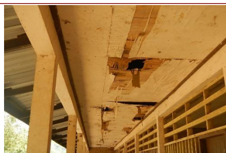
The main building is breaking down
