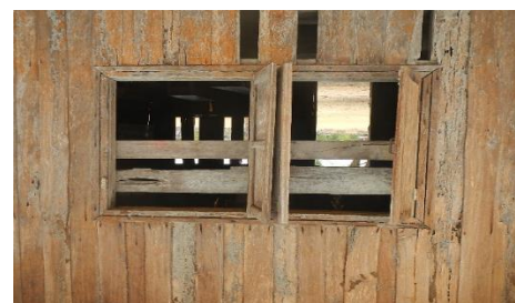
Termites have infested the wooden structures of the school building, rendering it unsafe for the students
