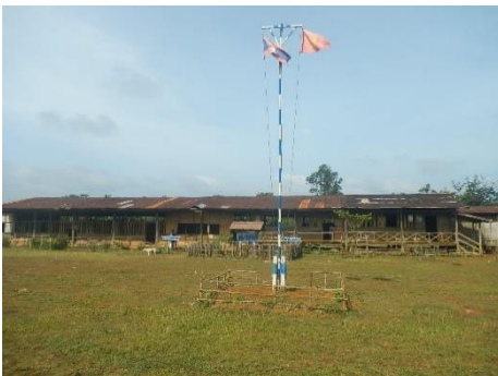
The wooden school building at Nong Pha Nuan Lower Secondary School is deteriorating fast and in dire need of replacement
