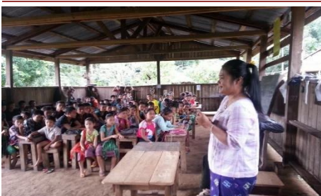
With virtually no walls, exposure to natural elements inhibits the ability of students to learn effectively
