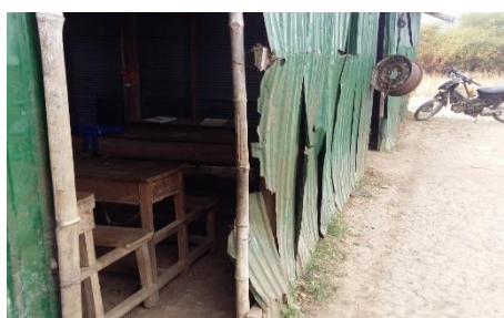
The walls are made out of metal sheets and its sharp edges are everyday risks to school children. The building is furthermore totally rotten.
