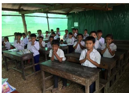
Primary school students attending class inside the rotten building
