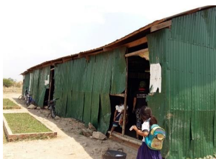
The temporary school building is deteriorating fast and in dire need of replacement
