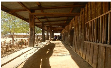
The temporarily school building doesn't provide a safe learning environment and is rotten.
