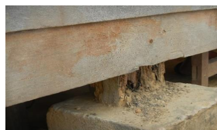
The building is deteriorating fast and might collapse anytime, potentially hurting children.
