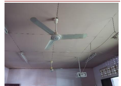
The existing projector and ceiling fans
