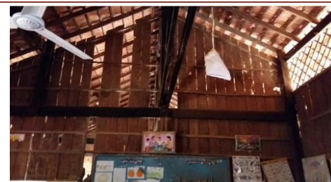
The existing, rotten O Khcheay Choeung Primary School
