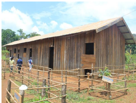
The wooden school building at Pha Nuan Dong Lower Secondary School is deteriorating fast and in dire need of replacement.
