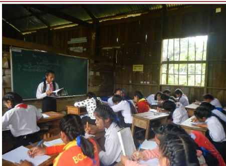
These classrooms offer inadequate protection against the harsh tropical weather. Furthermore, the building might collapse during a heavy storm.
