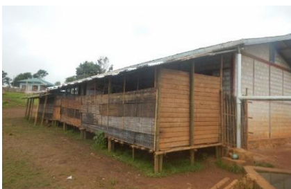
The temporary bamboo building is in very bad shape and needs urgent replacement
