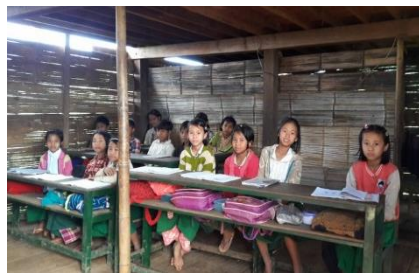
The walls of the bamboo building are rotten and have many holes
