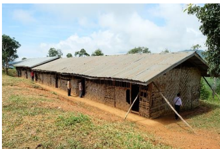
The school building does not provide a safe learning environment and has many holes in the walls
