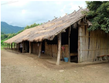
The school building does not provide a safe learning environment and has many holes in its walls
