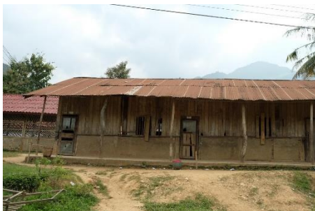
The school building no longer provides a safe learning environment and has many holes in the walls. Hygiene standards are very low.
