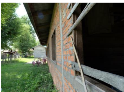
Poor construction of the unfinished building
