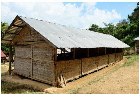
The rotten school building does not provide a safe learning environment for the students
