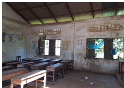
Dilapidated classrooms unsuitable for conducive learning conditions.
