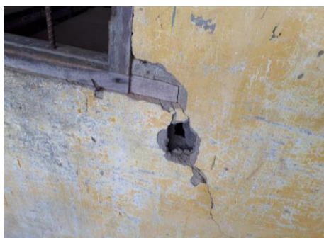
Walls and roof of the building are in very bad condition. There is risk the building could collapse.
