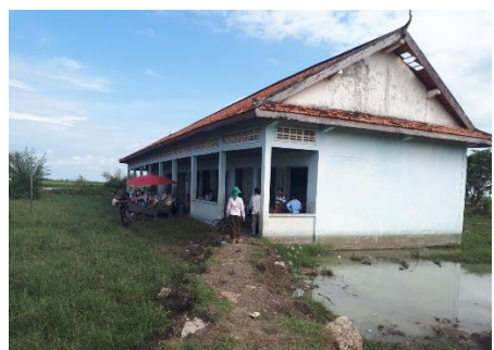
The rotten concrete school building amid the swamps and poor-conditioned grounds, unpalatable for pupils' recreations during their breaks
