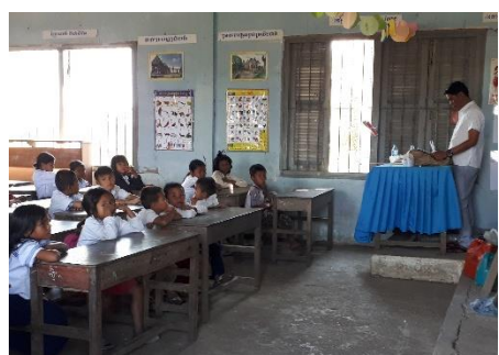
Inside one of the deteriorated classrooms with cracks around the building and the floor. This building might collapse anytime soon.
