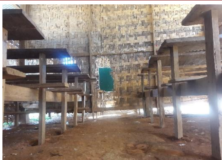
...and the walls of the thin bamboo woven panels are torn, exposing adjacent classrooms and noises of different lessons, resulting in distractions.
