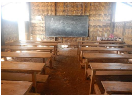
The inside of a classroom in one of the bamboo buildings, very much lacking in decent resources...
