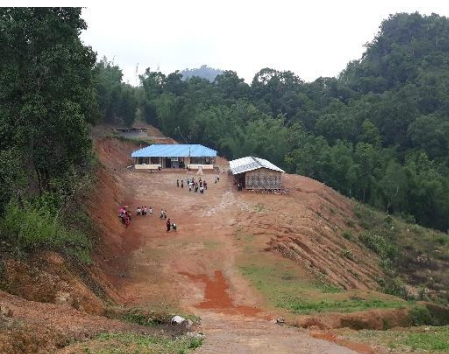
The temporary bamboo building (on the right hand side) has woven bamboo walls and a zinc roof. It is in dire need of replacement.
