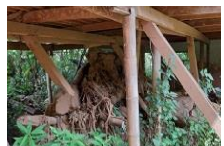
Deteriorating building foundation
