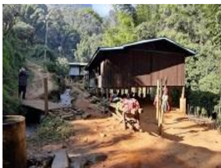
One of the existing, rotten school buildings
