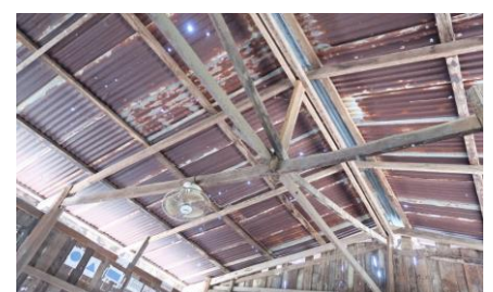
The rainwater gush through the holes in the roof, causing intense structural damage. The building can collapse anytime soon.
