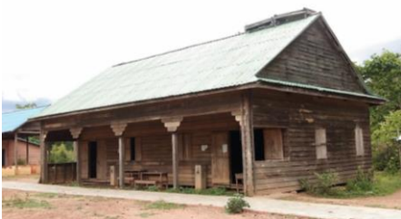
One of the old, dilapidated schools buildings
