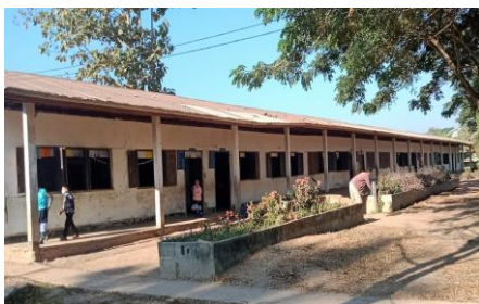
The old, earthquake damaged primary school building must be demolished and replaced
