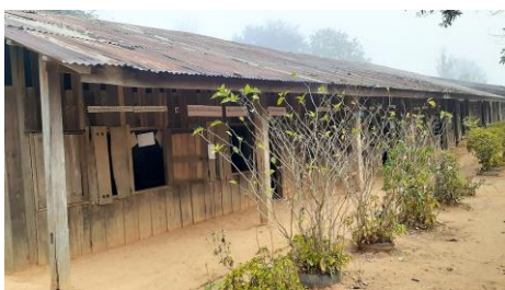
The old, dilapidated school buildings are in dire need of being replaced
