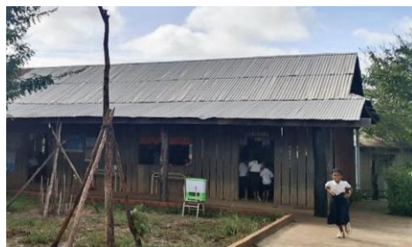
The dilapidated school building will be removed
