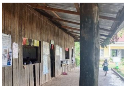
Old, rotten wood with clear signs of deterioration
