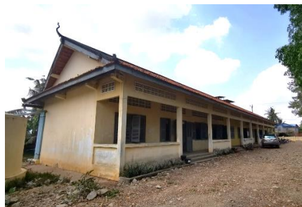
Phkam High School is in reasonable condition, but lacks a functional computer laboratory
