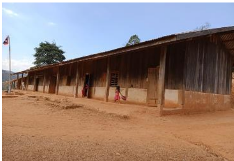
While the oldest of the three buildings is still structurally safe, it is nonetheless in poor condition.
