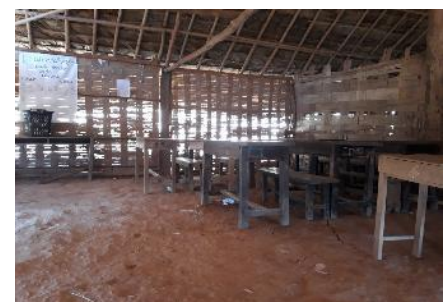
The gaps in the walls and roof allow rainwater in, causing the dirt floors to turn to mud.
