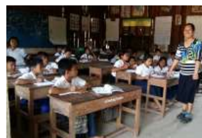
The walls in the classrooms have large holes, allowing rain and noise to enter, creating a chaotic and unproductive learning environment
