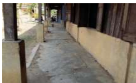
The other building, consisting of rotten wood and a cracked concrete base, poses a great safety risk to the students who learn in it
