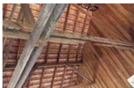
The wooden roof trusses are rotten and on the verge of collapse
