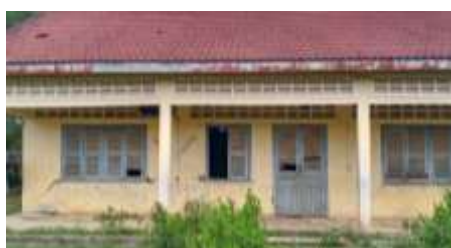
One of the concrete buildings is so severely cracked that students are no longer allowed to enter it
