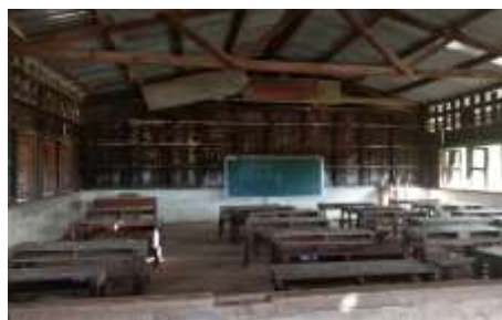
The integrity of the buildings presents severe safety risks to the students and teachers
