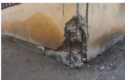
The metal rods are exposed and don't offer adequate support
