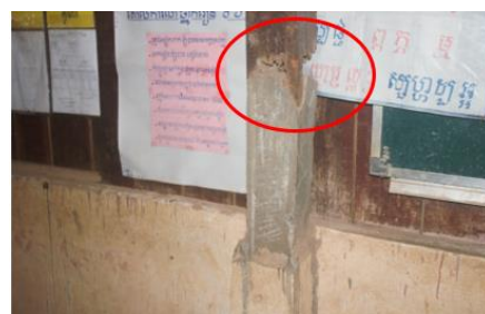
The support beams are rotten and could collapse without warning
